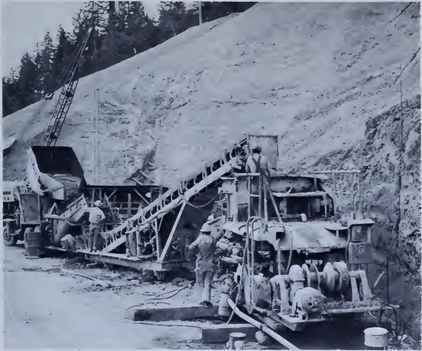
Figure 134.—Equipment and method used for pumping concrete into spillway tunnel at Trinity Dam, Central Valley project, California. TD-5008-CV.
